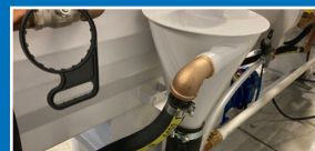
Vacuum pump discharge water air separator
